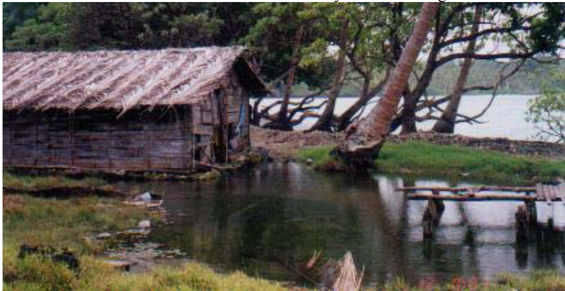
Plate 2 House materials rot easily due to flooding
