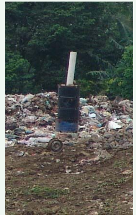
Above: One of the vents in the landfill, giving off less harmful CO 2 and passively sucking air into the pipes for aerobic garbage / leachate breakdown.
