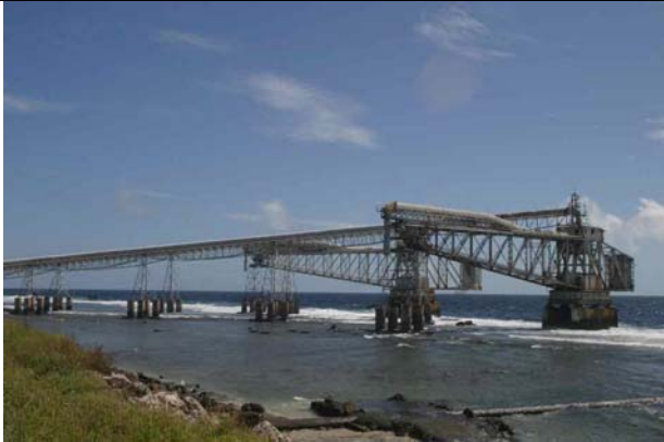
Figure 1-6 – Phosphate Cantilevers for Ship Loading
