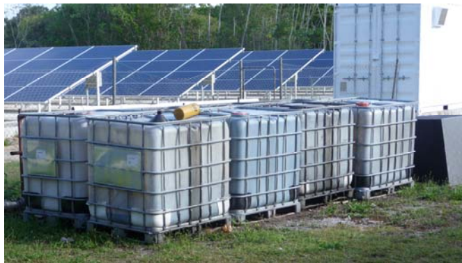
Temporary storage at the Niue power generation site
