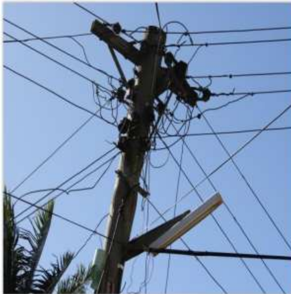
Poor condition of wiring and power poles in Nuku'alofa
