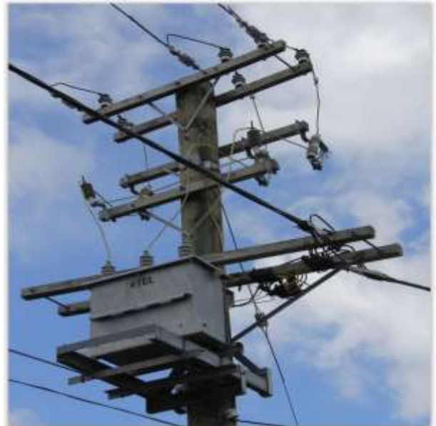
Recently upgraded power poles and lines
