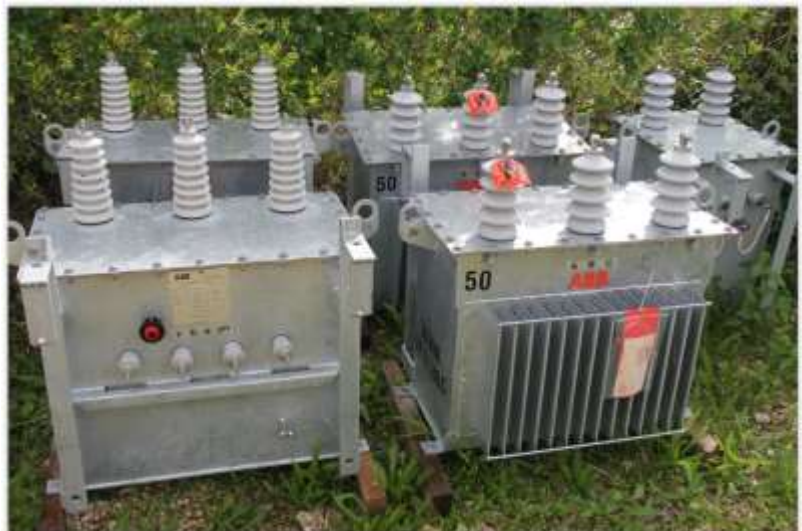
Photo 8: Distribution Transformers in TransNet Store
