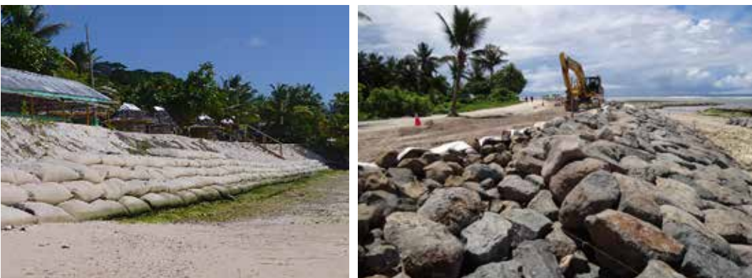
Figure 3-3 Semi-Rigid Geotextile Container at Manase, Samoa and a Rock Revetments on South Tarawa, Kiribati
