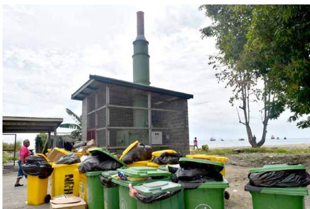
FIGURE 7.11. Large Incinerator installed at National Referral Hospital in Honiara under the SPREP PACWASTE Project (© Allen Kisi Ofea/ECD 2017).
