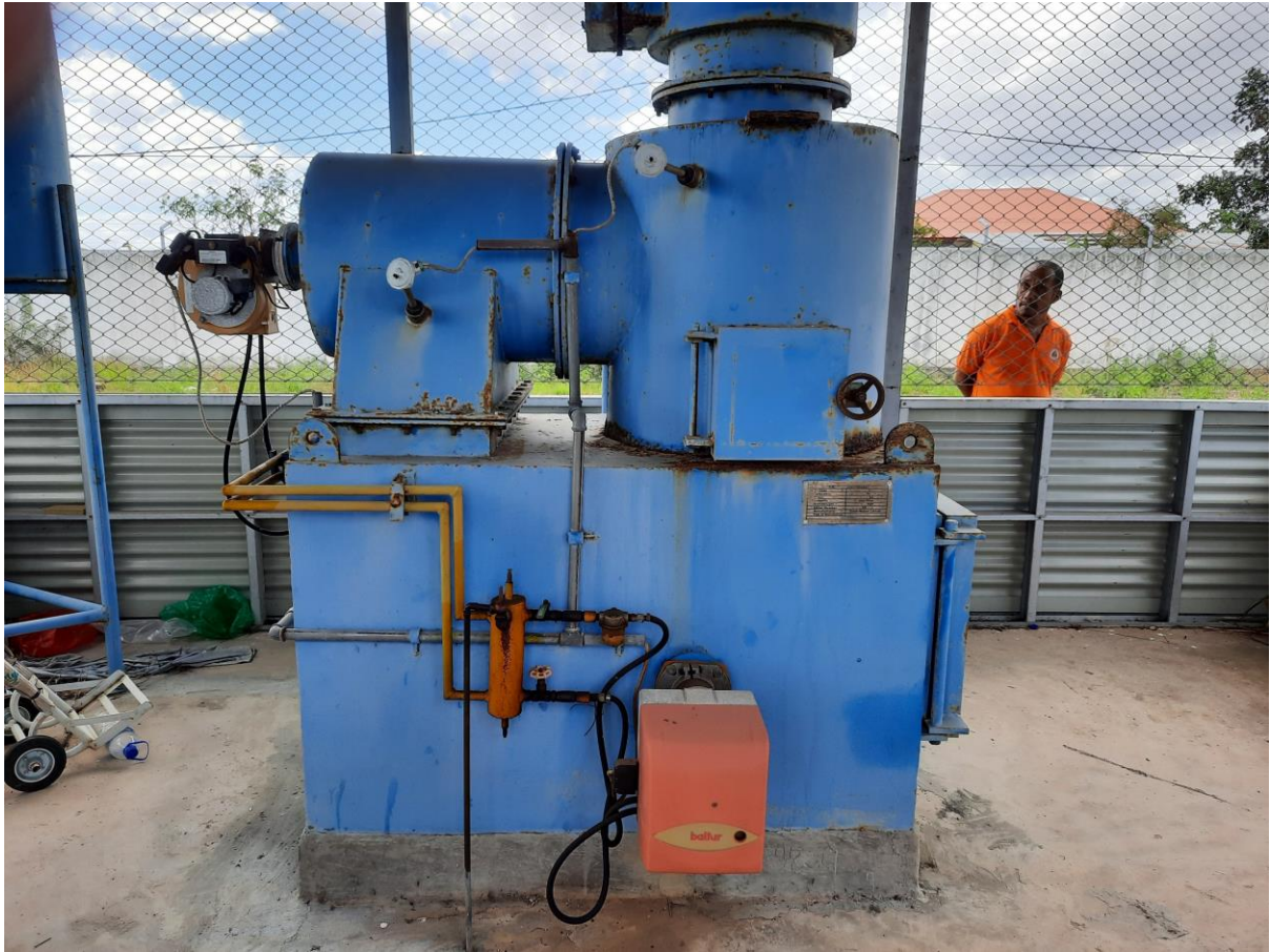
Figure 4: Hospital East Incinerator [Chinese funded], Baucau Hospital, Baucau, Timor Leste, August 22, 2022, Photo taken by Lance Richman
