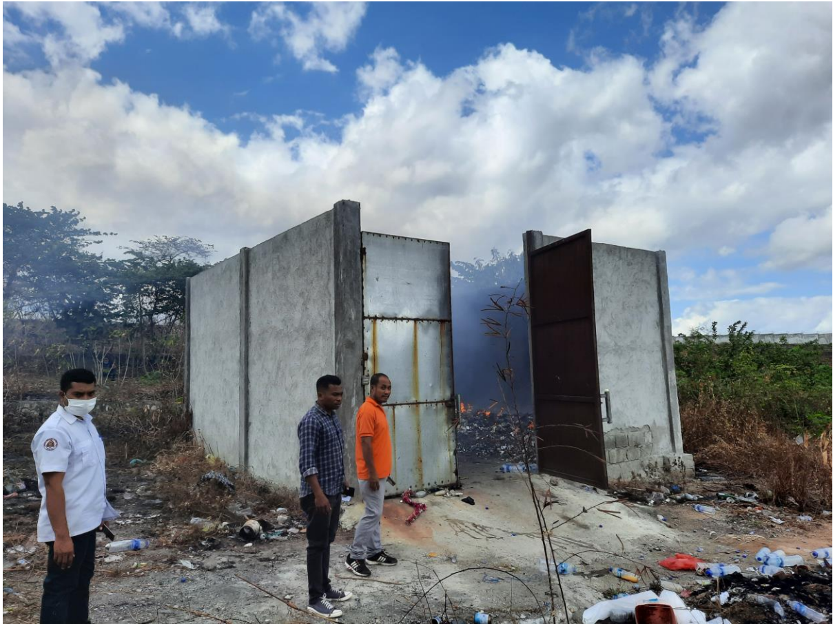
Figure 3: Hospital West Burn Facility [WHO funded], Baucau Hospital, Baucau, Timor Leste, August 22, 2022, Photo taken by Lance Richman
